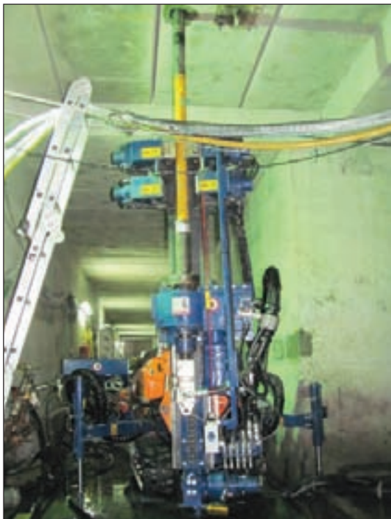
The Comacchio MC 3 D unit working in low-overhead conditions inside the galleries
